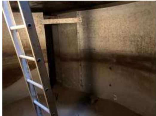
Inside sediment vault
