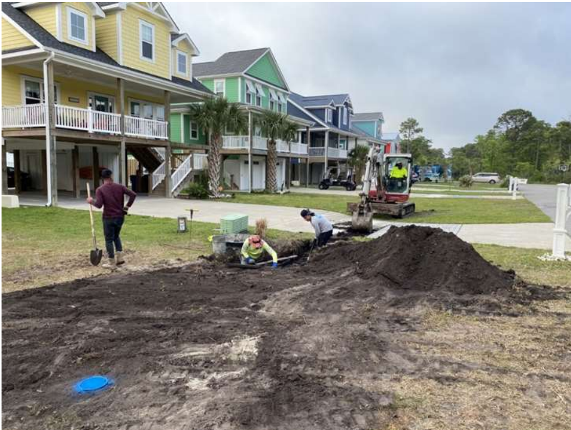
Contracted crews begin work installing stormwater drainage on the 1400 block of Croaker Lane.
