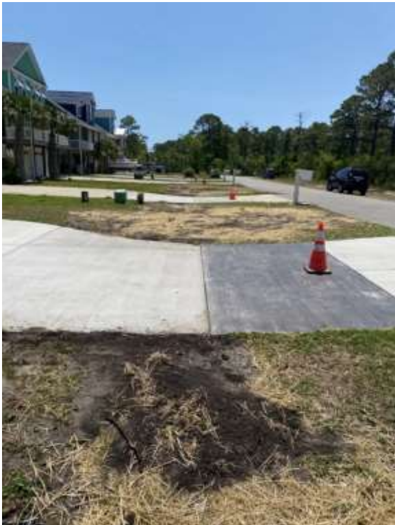
Contracted stormwater project at Croaker Ave is complete. Five basins installed four driveways removed and replaced.
