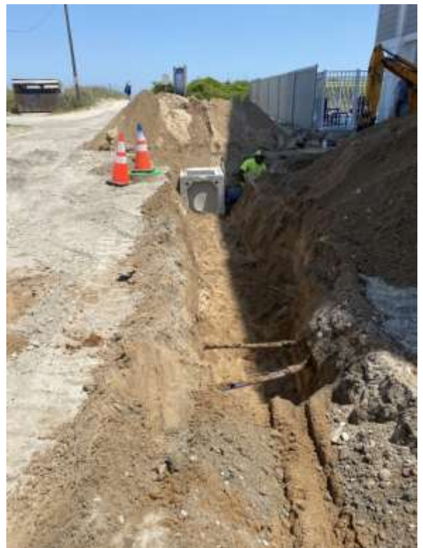
Contracted services to add stormwater to Hamlet Ave. beach access have started and are expected to be completed soon.
