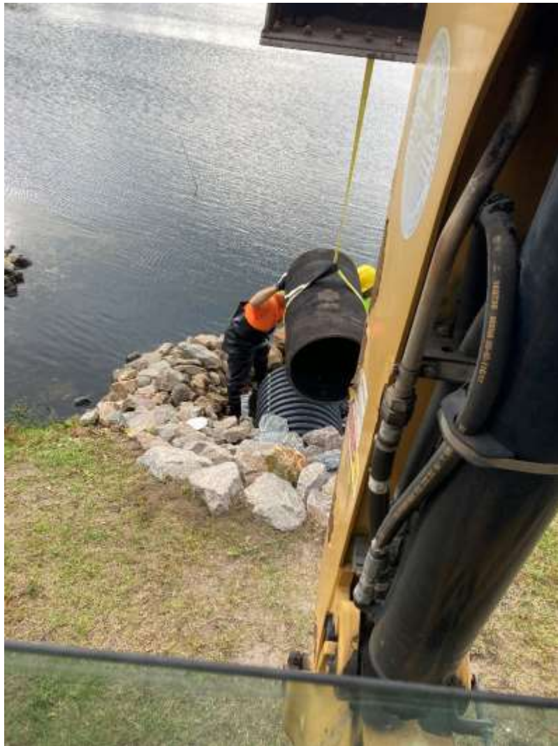
Crews install a check valve at the Lake to help prevent stormwater backflow into the neighborhood.
