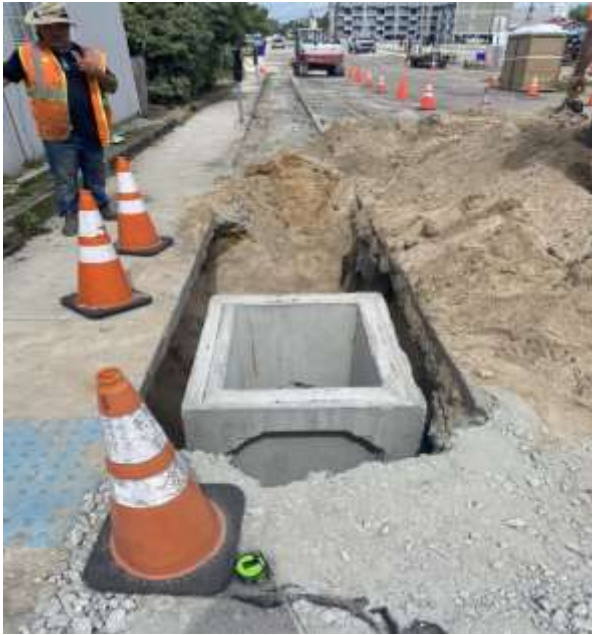
Contracted crews continue adding stormwater infrastructure from CBAS to Woody Hewett Ave.
