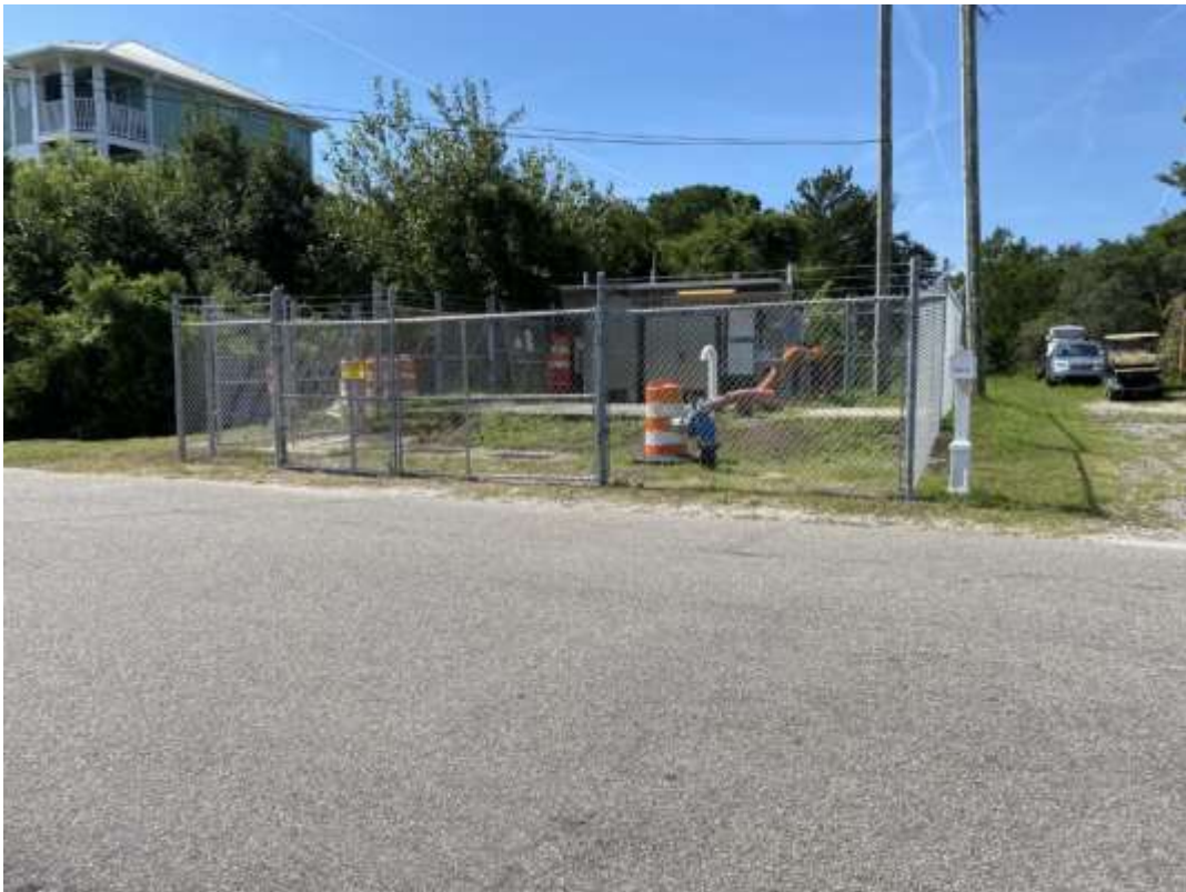
Contractors added security fence to Greenville Ave. and 2 nd street pump facility; privacy slats will be added.
