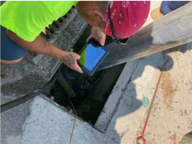
Crews trained on video equipment to record the conditions of underground pipe.
