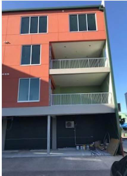
REAR VIEW (SEE ALSO LOW HVAC) TAKEN 04/22/20
