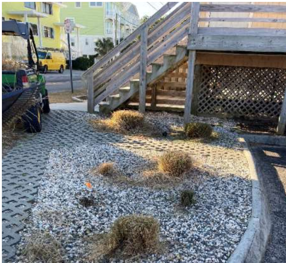
Crews trim back vegetation and renew stormwater drain beds at the CBA North public bathroom.
