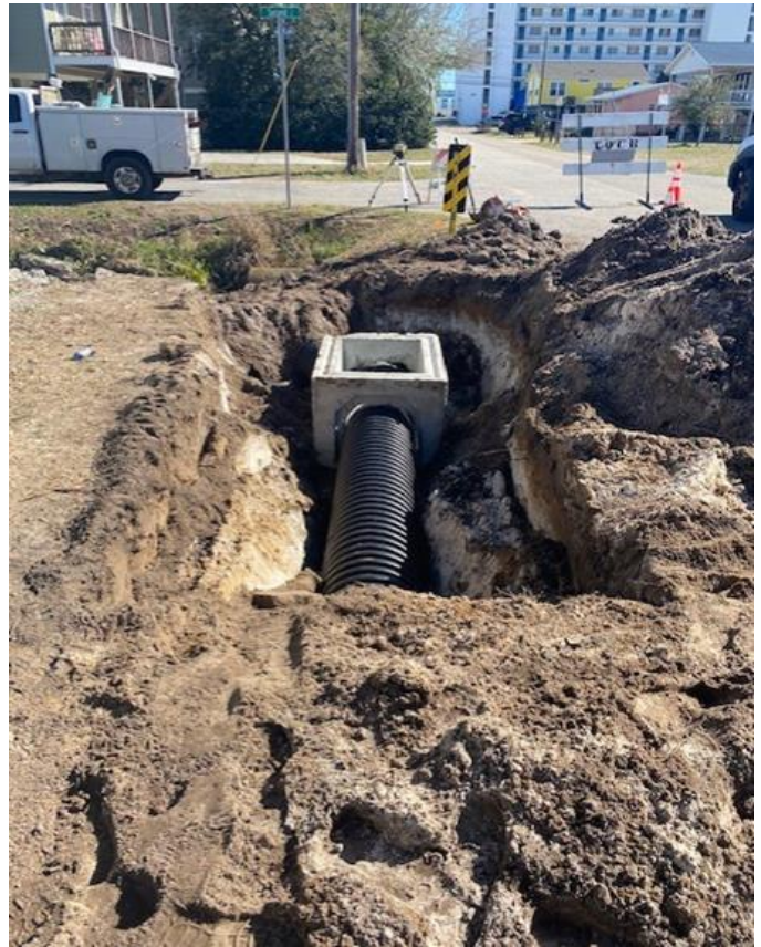
100 Contracted work to upgrade the stormwater systems on Spartanburg Ave have begun.
