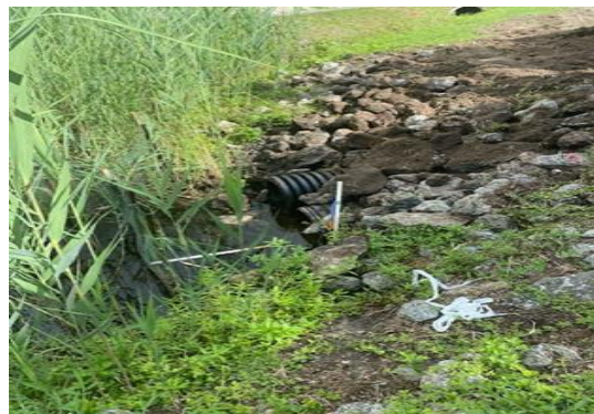
Contractor installed additional stormwater pipe under the 1100 block of Saint Joseph St.
