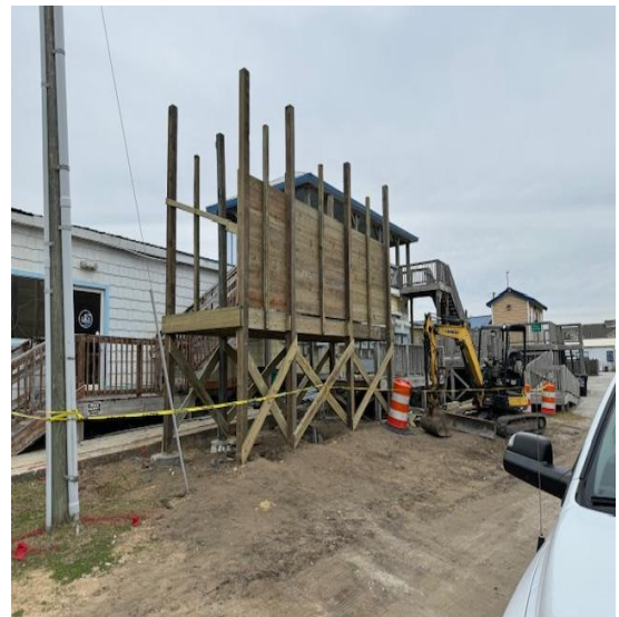
Electrical platform in CB Municipal Marina
