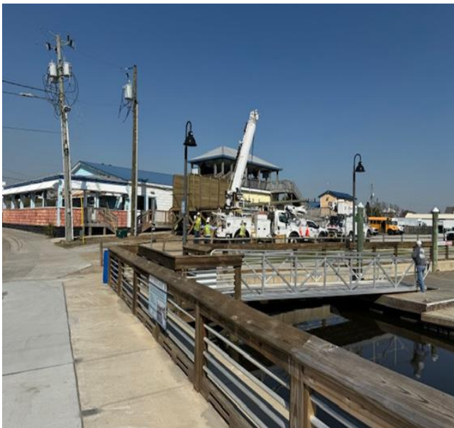
Marina Project: Duke Energy removing power Pole to make room for new electrical platform.
