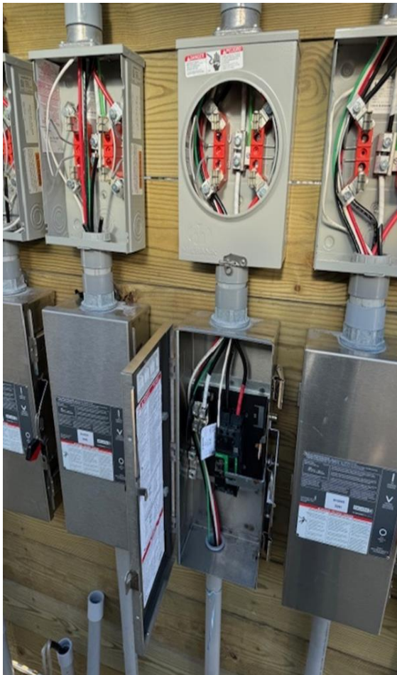
Power connections from dock pedestals to meters installed
