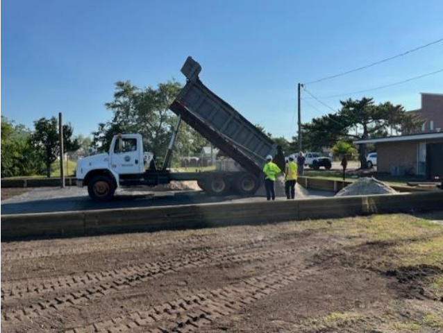
Stormwater crews haul sand for the new volleyball court on Cape Fear Blvd.
