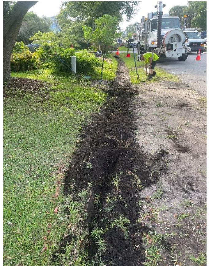
Stormwater crews continue working to re-establish ditch on 500 block of Greenville Ave.
